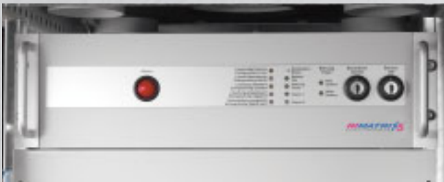
Extinguisher systems with smoke extraction
